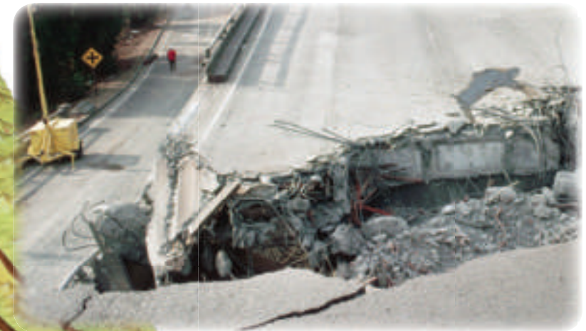
An earthquake damaged this road.
