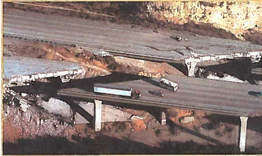
▲ Route 14 near Sylmar, California, was heavily damaged as a result of an earthquake on January 17, 1994.
